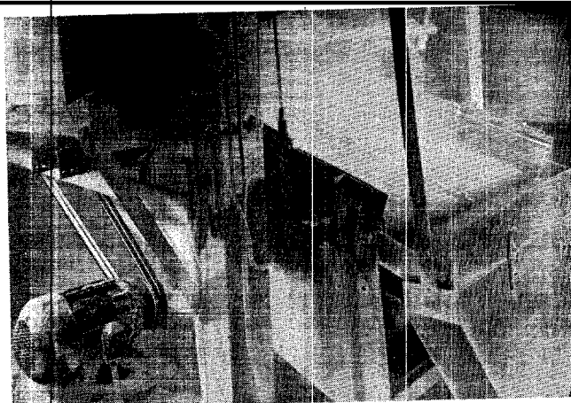
Fig. H-30. Dust in lime plant dictated selection of this 7½-hp, totally-enclosed fan-cooled motor.
