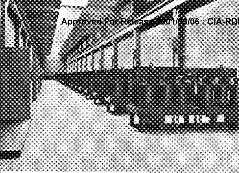
◀ 120,000-ampere, 673-volt Ignitron Rectifier installation for electrochemical service.
