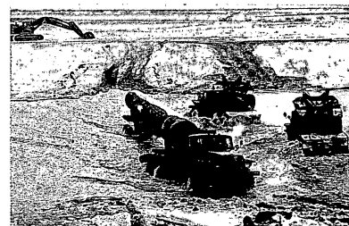
Pipe sections are transported by trucks from railyards to the construction site.
